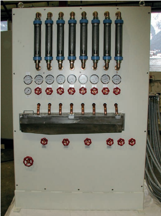
Cooling water control and connection unit with open cooling water circuit
