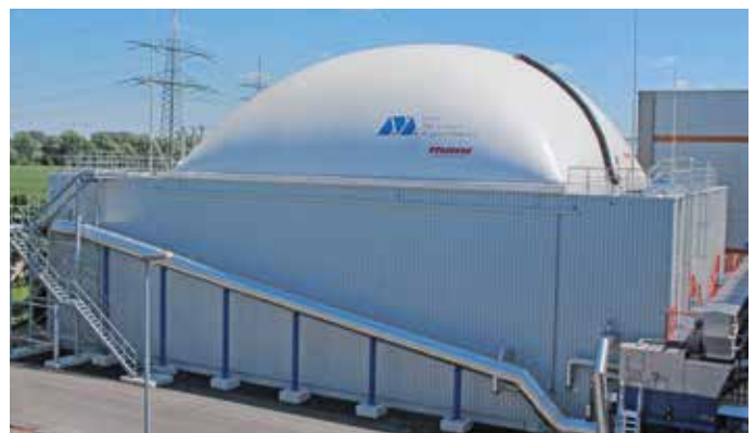
Biogas plant with gas storage unit
