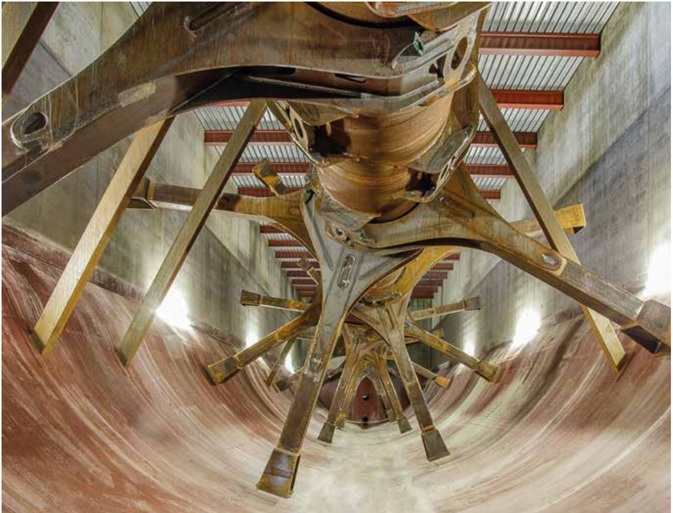
TTV digester - internal view
